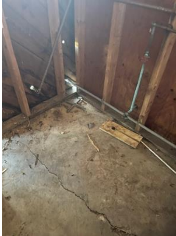
CONDITION OF SLAB
