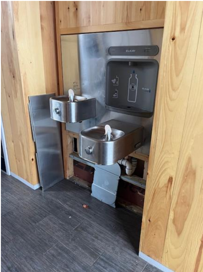
ACCESSIBLE WATER FILLING STATION
